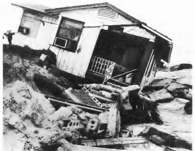
Figure 2.3. Erosion Caused This Foundation to Collapse.
