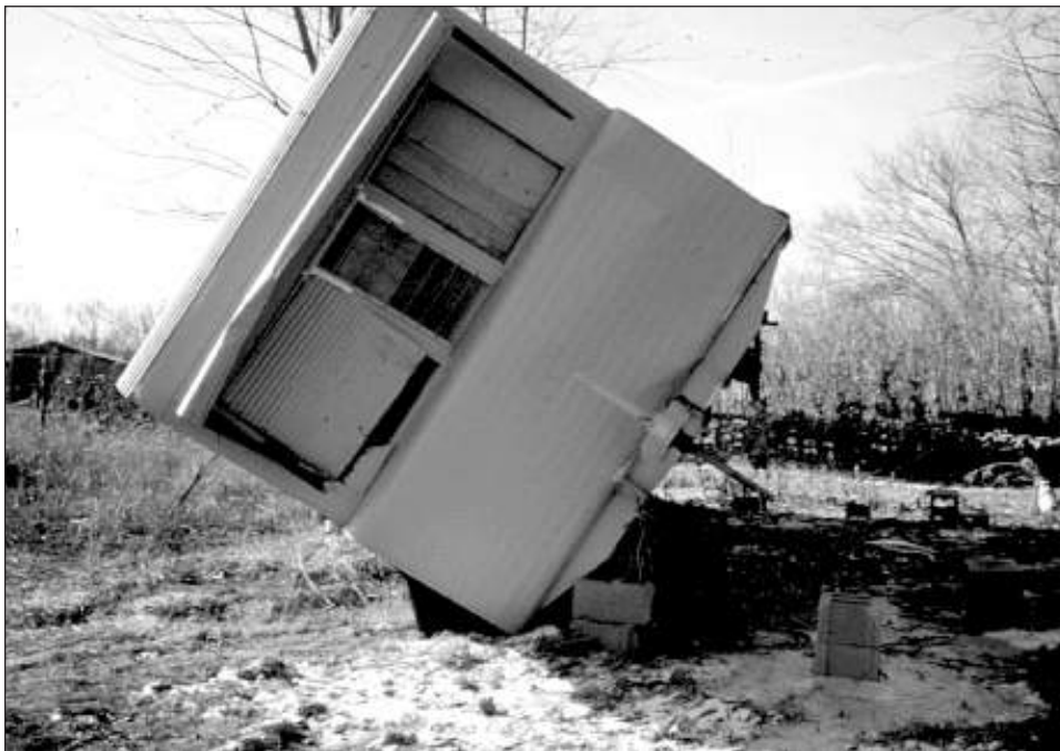
Figure 7-8. Failed foundation system that used masonry piers.
