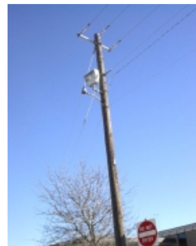
Typical Utility Pole with Floodlight
