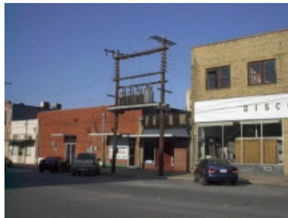
Existing overhead transformers should be replaced with a pad-mounted fixture on the ground, as utilities are placed underground.
