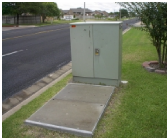
Pad-mounted electrical transformers will appear as overhead utilities are placed underground. Placement of these pad-mounted fixtures will need to be carefully planned to occur in areas where they can be screened effectively.
