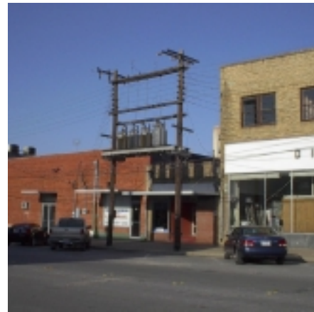
Overhead utilities are currently prevalent within the core study area, especially on Bryan Avenue.
