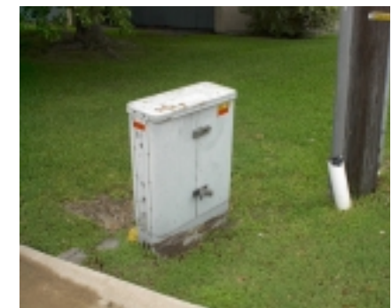
Communications pedestals and pad-mounted electrical transformers will appear as overhead utilities are placed underground. Placement of these pad-mounted fixtures will need to be carefully planned to occur in areas where they can be screened effectively.
