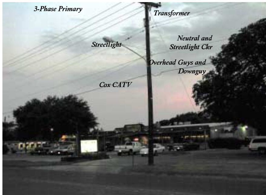
Figure 7.1 - Typical Utility Pole on South College Avenue
