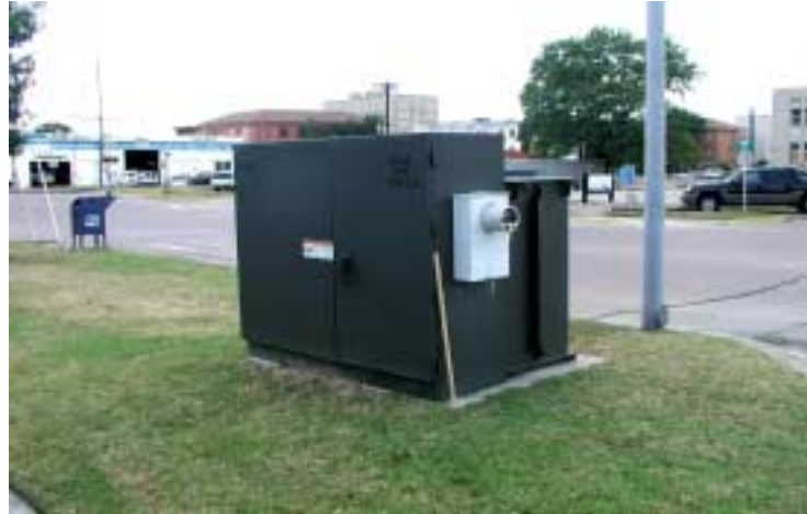
Figure 7.2 - Three-phase Wye Pad-mounted Transformer
